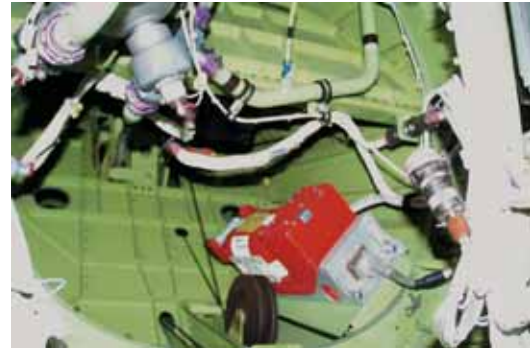
Figure 14a—Tailcone Interior Open and check for: fluid leaks, main engine fire bottle pressure, security and condition of installed equipment; remote circuit breakers—set; APU (if installed) fire bottle pressure and APU FAN FAIL indicator; condition of door seal, then close access
